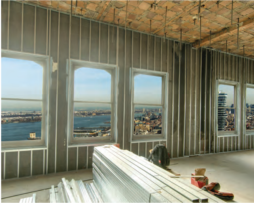
The physical anchorage of an aluminum window is critical to ensure that it performs and operates as designed and tested. Photo credit: Oleg March and Travis Mark.
