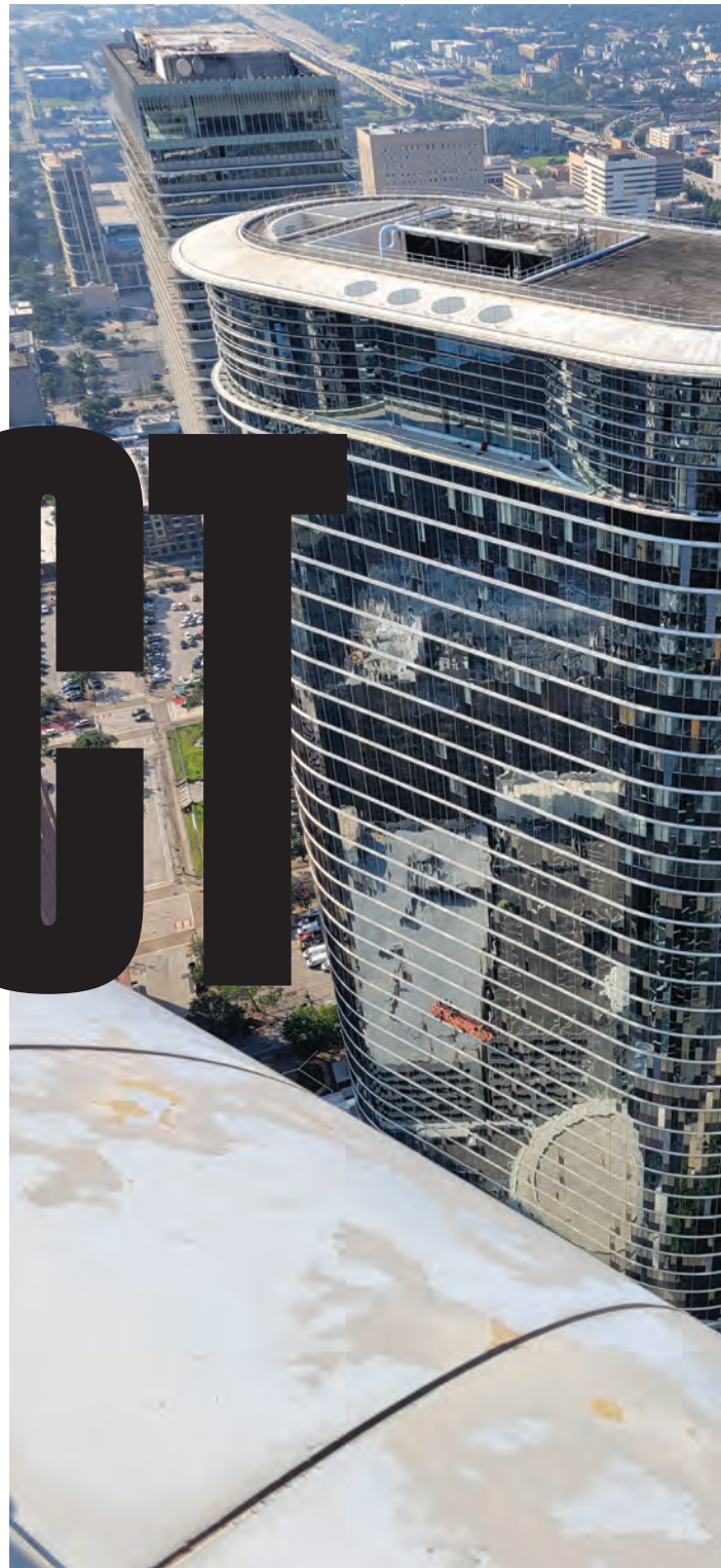
COMMERCIAL OFFICE BUILDING IN HOUSTON, TEXAS, DAMAGED BY STRONG WINDS.
